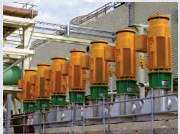
Duplex SS Seawater pump for Nickel Mine
