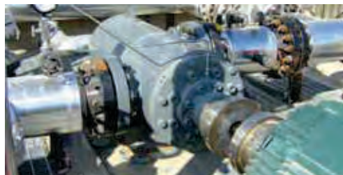
4 Crude Transfer Pump L3MG
