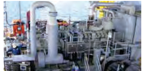
1 Multiphase Pump L4HK on an Offshore Platform
