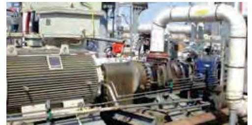
2 Pipeline Start-Up Pump L4HK
