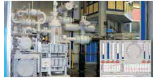
Leistritz Multiphase Pump system on the Test Field
