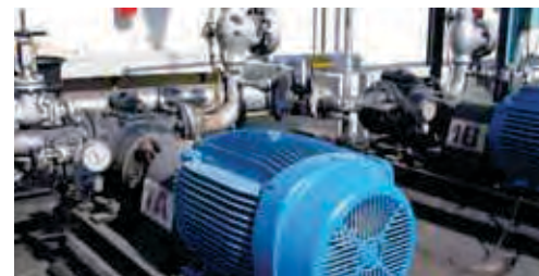
4 Slops & Drains Oil Pump L2NG
