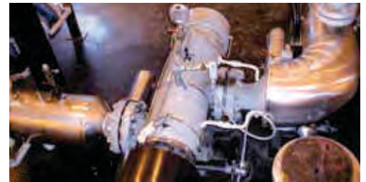
1 Crude Circulation Pump L3HG
