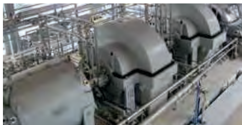
1 Compressor Lube and Seal Oil Pump L3
