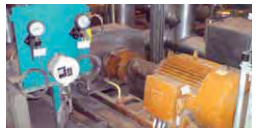
4 Crude Stripping Pump L4NG
