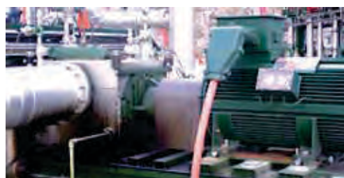
1 Unloading Pump L4MG
