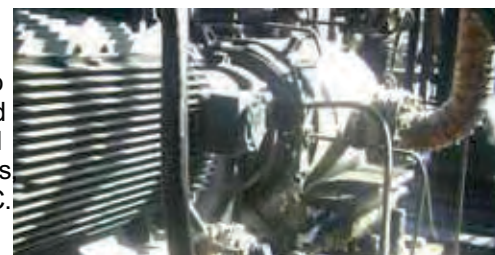
3 Vacuum Residue Pump L4MG
