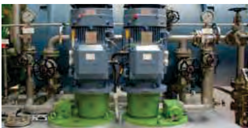
2 Auxiliary Lube Oil Pump L3MF
