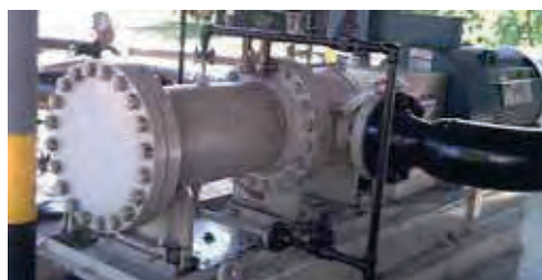
3 Crude Booster Pump L3HG
