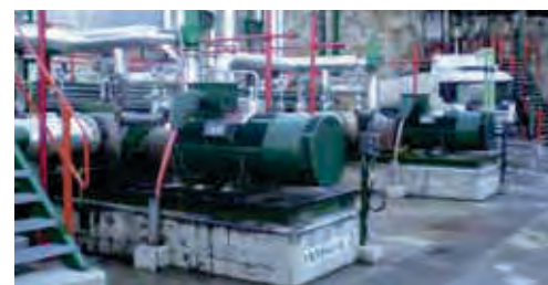
2 Crude Charging Pump L4NG
