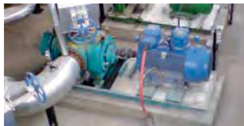
4 Stripping Pump L4NG
