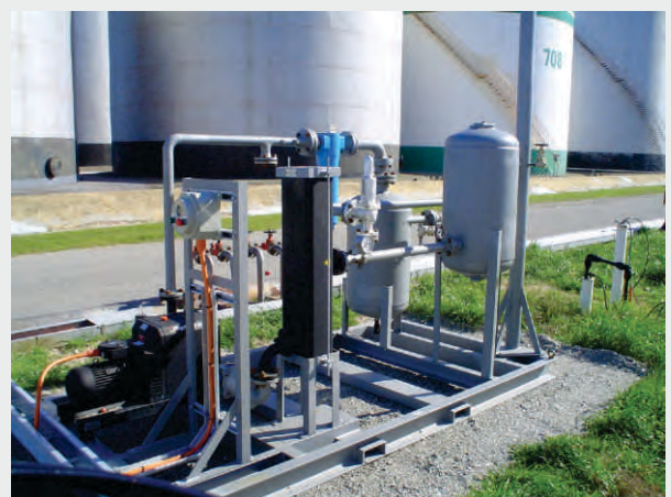
Claw Type Vacuum Pump Skid on site in Kwinana, WA
