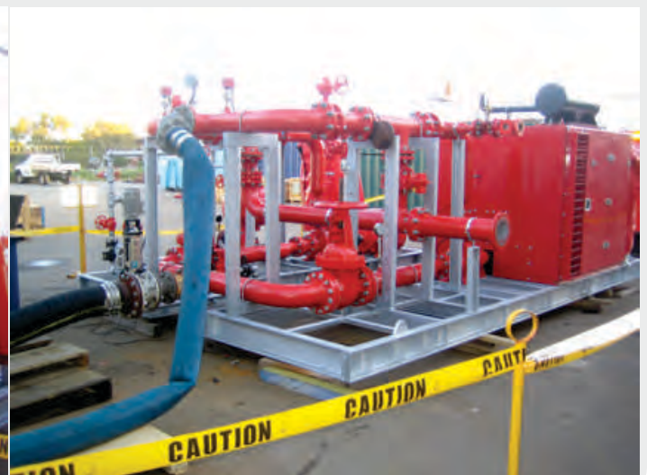
Fire Water Pump set undergoing performance and functional testing
